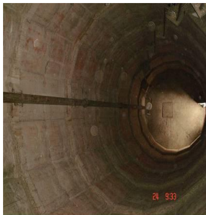
FIGURA 48: INTERIOR BASE TANQUE
