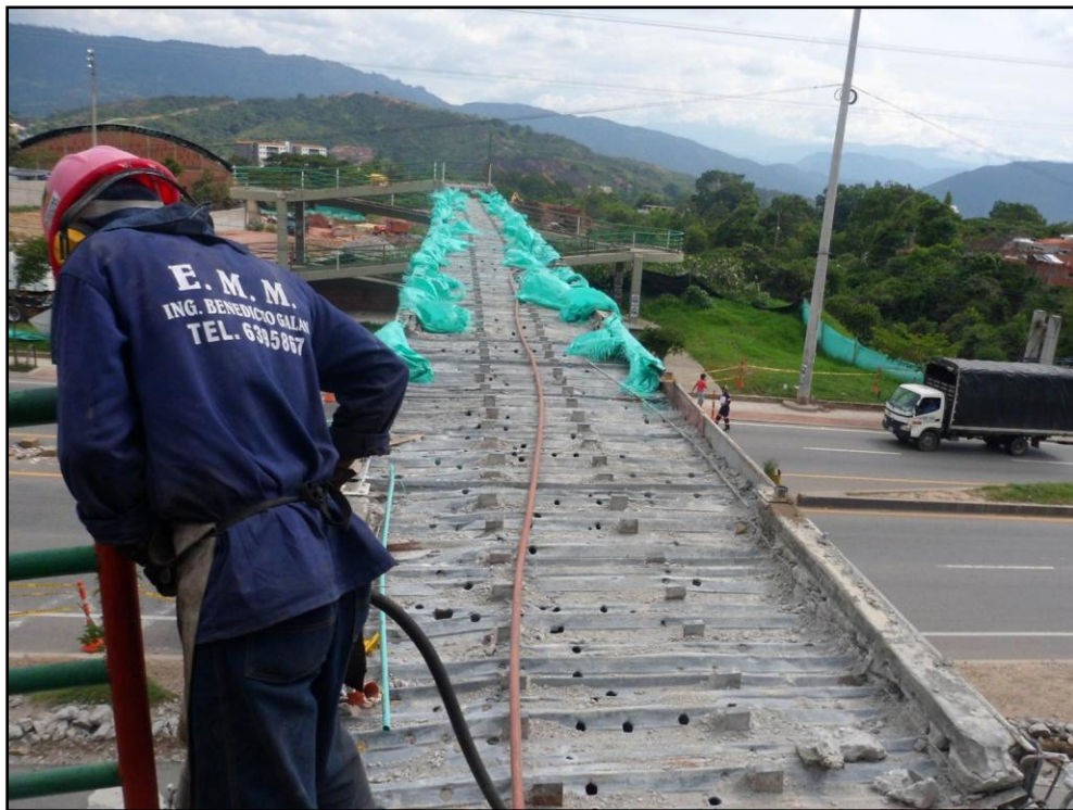
Figura 42. Tablero principal sin concreto
