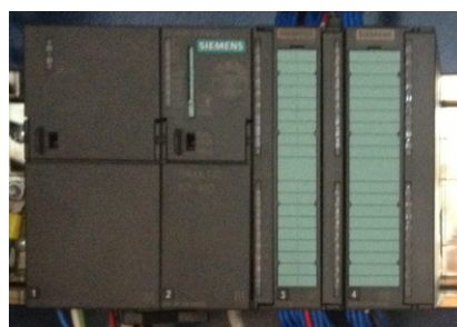
Figura 3.4: PLC S7-300 y módulos IO
