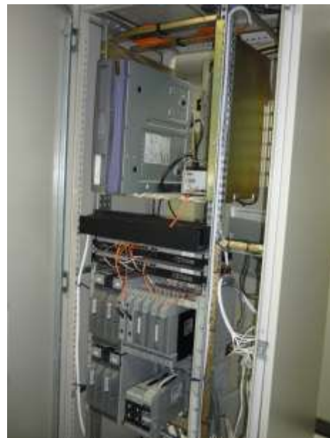
Figura No. 53 Gabinete E22200
