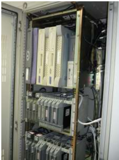
Figura No. 52 Gabinete E22701
