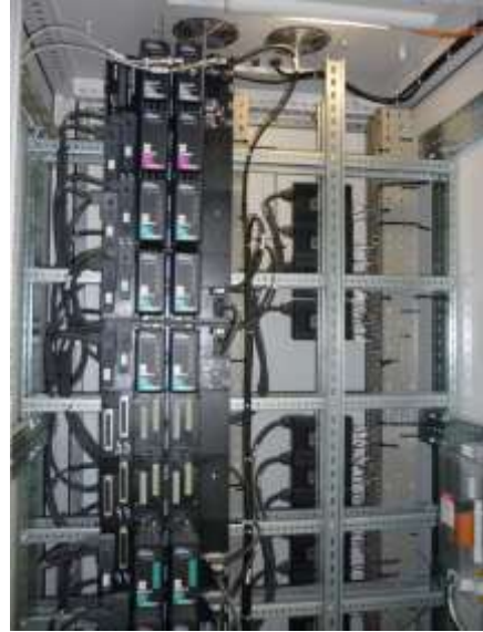
Figura No. 47 Gabinete E22001
