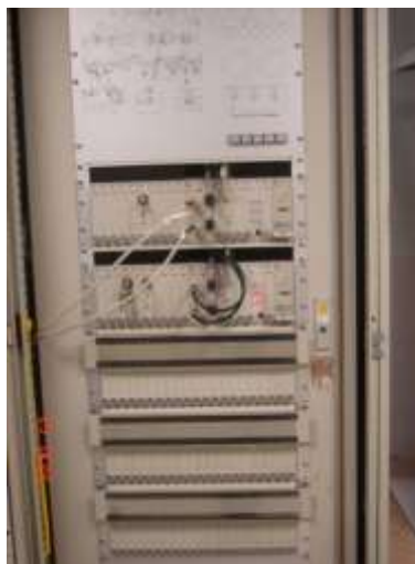
Figura No. 68 Gabinete E13000
