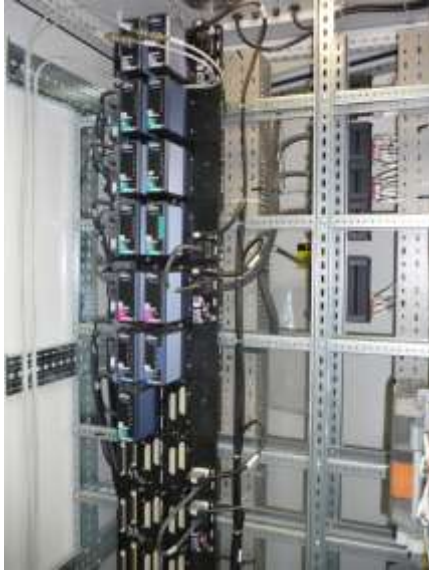
Figura No. 46 Gabinete E22000
